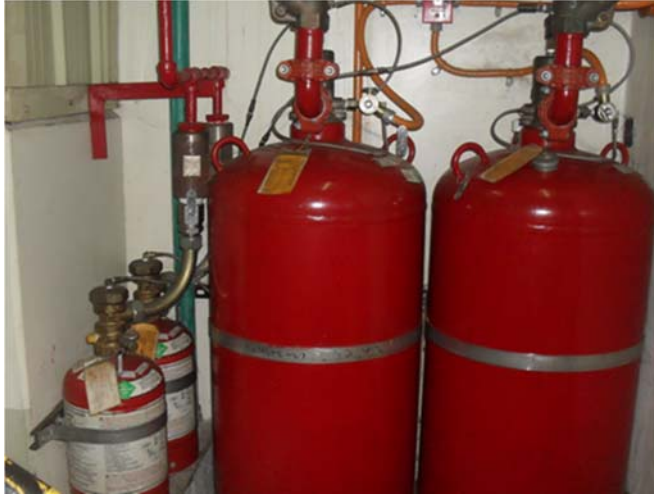
FM-200 Fire Suppression System
