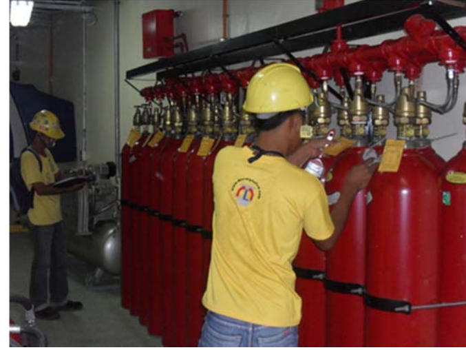
CO2 Fire Suppression System
