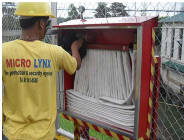
Fire Hose System
