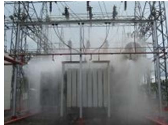
Deluge Water Spray System
